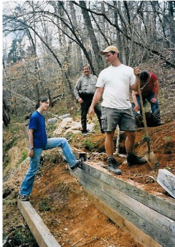
Lori Davias and Edward Malindzak stop to admire their work. Several students built a retaining wall and planted trees along the Eno River to stabilize the bank.
