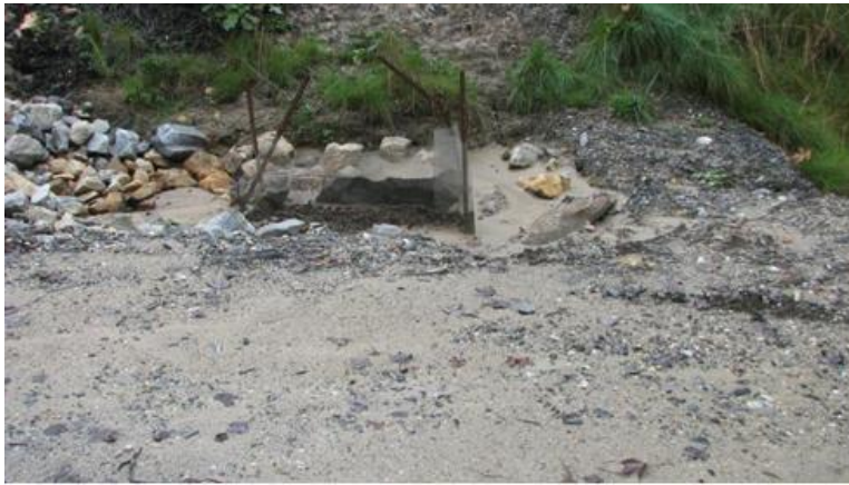
Failed sediment screen on a road cross drain inlet in the brook trout stream watershed, September 2009.
